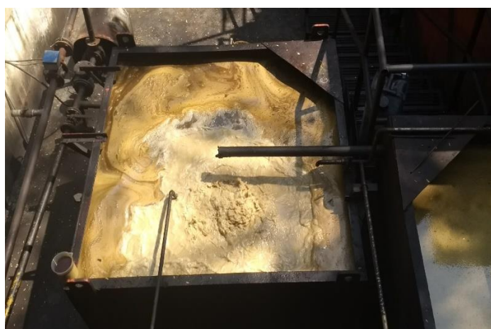
Figure 8: Acid Addition at the coolant storage tank
