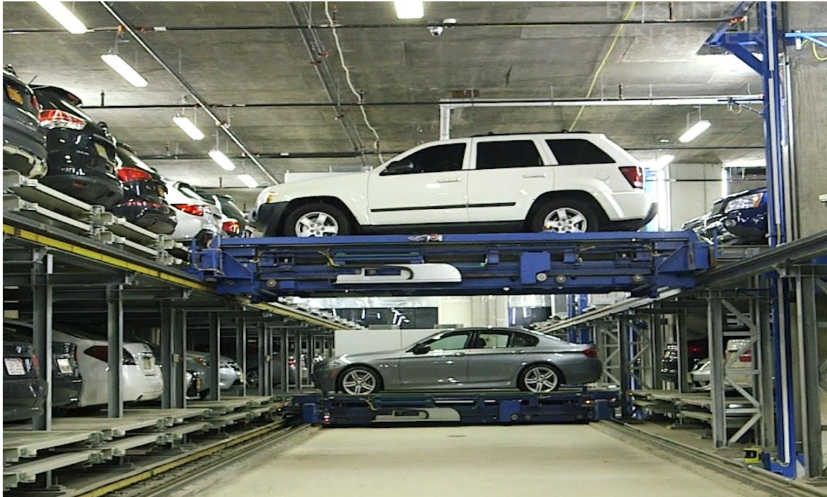
Plate 10. Automate Parking system in Liverpool
