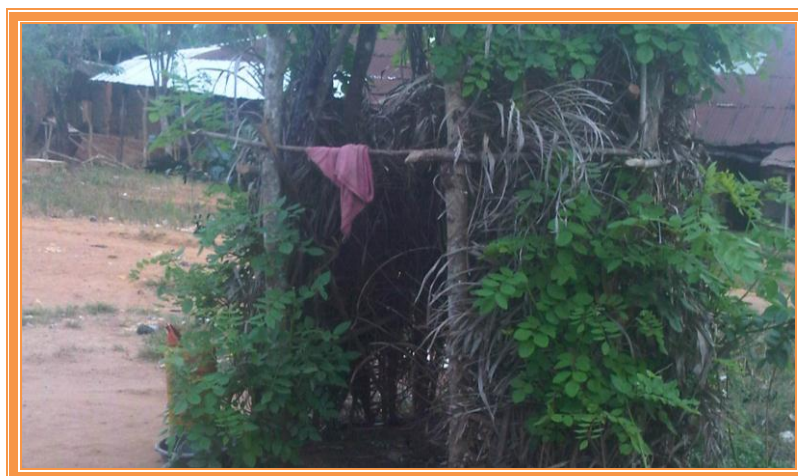
Fig. 2. Condition of an External Bathroom in Abata-Egba
